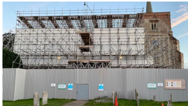
Scaffolding on the North side and over the nave roof during the building works - St Leonard's, September 2021
