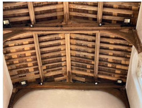
The nave roof timbers; no attempt was made to colour the new wood to match the old; December 2021
